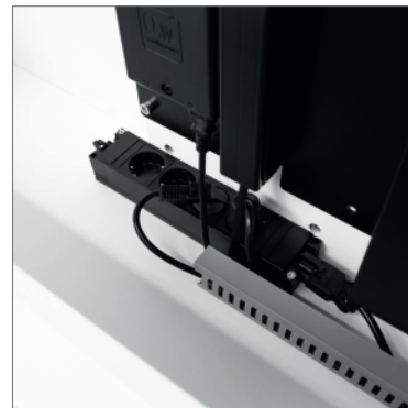
Fig. 3 Multiple outlet sockets
